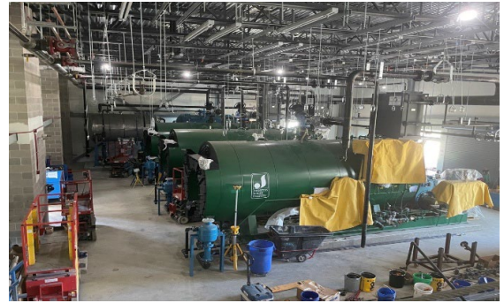
New plant at Elgin Mental Health, interior view. Elgin.
