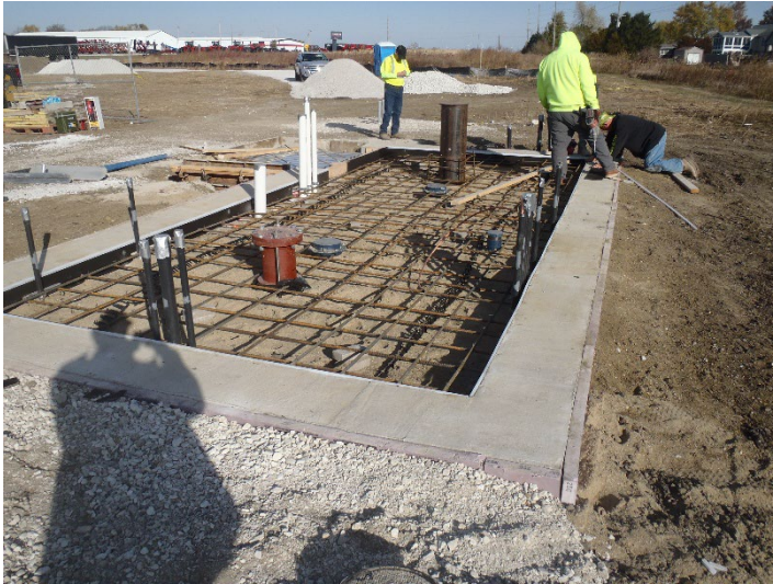
New well and water treatment plant improvements. Gibson City.
