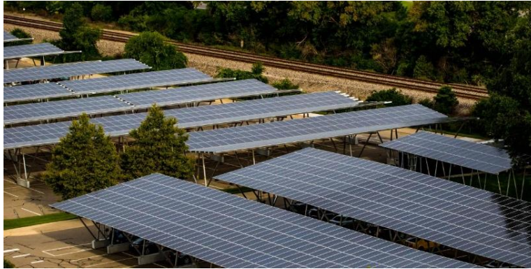
Solar canopy above surface parking lot.
