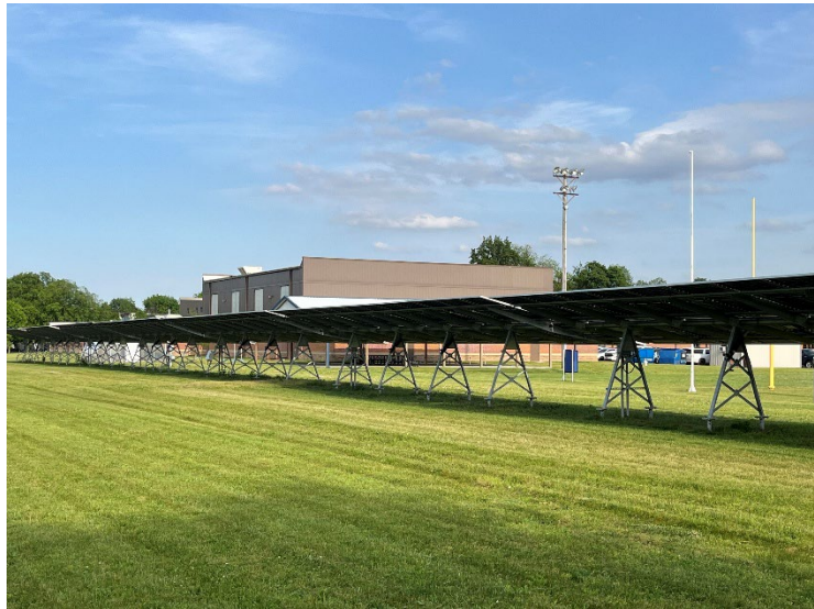
On top of its financial benefits, Palestine School District’s 129.6 kW solar project serves as a hands-on opportunity for student to learn about solar technology and the power of the sun.
