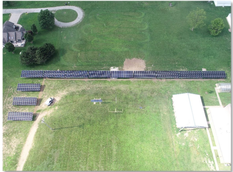
Illinois Shines Public School Category solar installation at Palestine Grade School.
